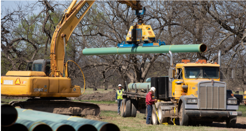
Workers at a site of a pipeline under construction along state Highway 75 north of Horntown. (Photo by Brent Fuchs)
